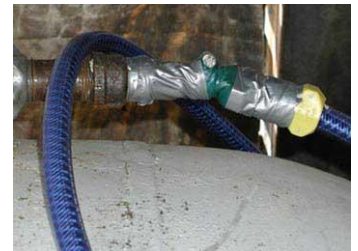
Homemade pipe fittings on tanks or thermoses
