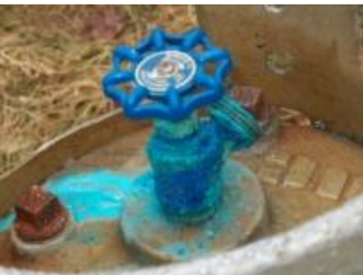
Propane tanks with painted or corroded brass fittings. Suspect propane tanks often have a bluish-green coloring
